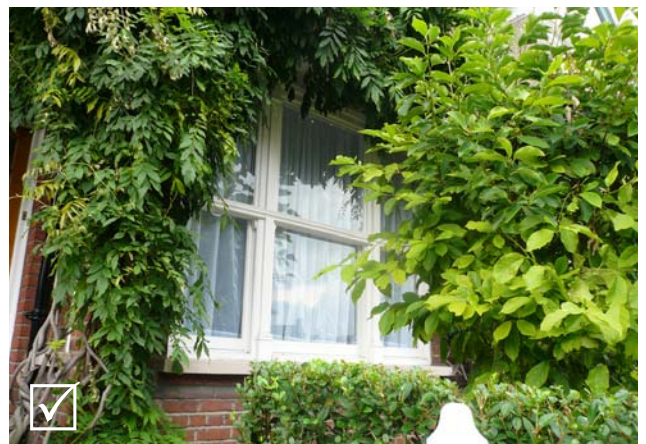
Fig 6.2: Traditional windows can be effectively refurbished and maintain key characteristics of the property
