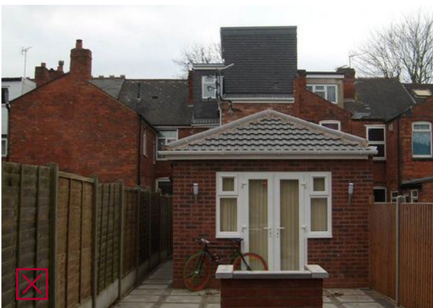
Fig 4.12: Poorly considered infill extensions can result in left over, narrow, external "corridor" spaces.
